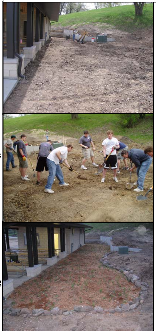
PHOTOS: Whitewater “Make a Difference Day” and UW-Whitewater Freshmen for Freshwater rain garden project, Spring 2010. Before (top), during construction (middle) and after (bottom).
